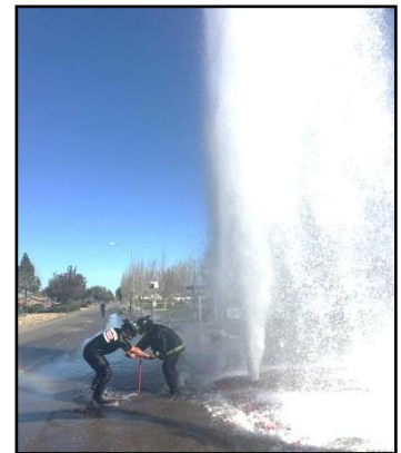
Manteca firefighters turning off the water to the damaged fire hydrant.
