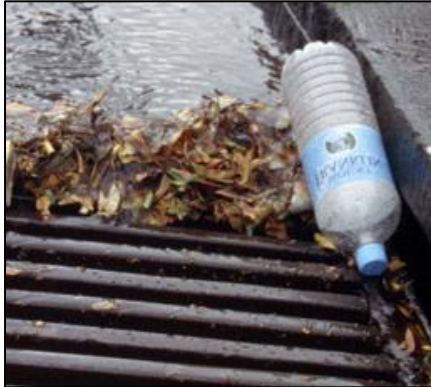
Garbage that has made its way to the storm drain.
